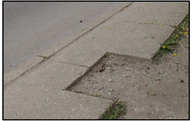
Photo 1: Missing Sidewalk East of Dollar General
