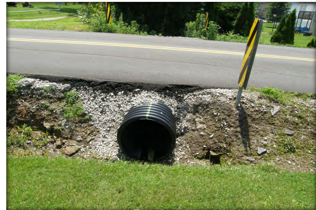
Figure 6: Existing 24" HDPE West of the Mount Vernon Baptist Church (Looking South)
