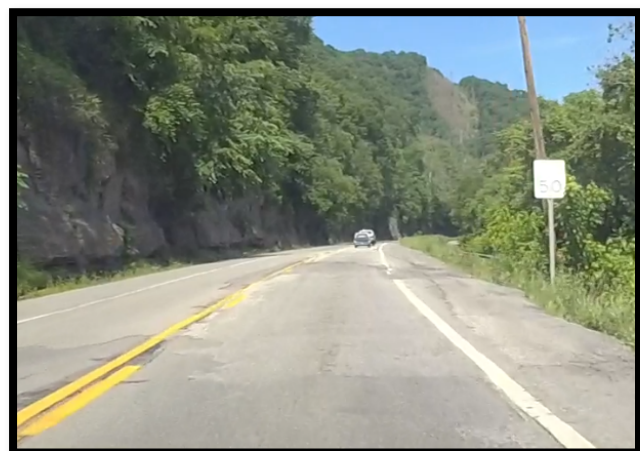
Photo 1: Washed Out Pavement on US 60
