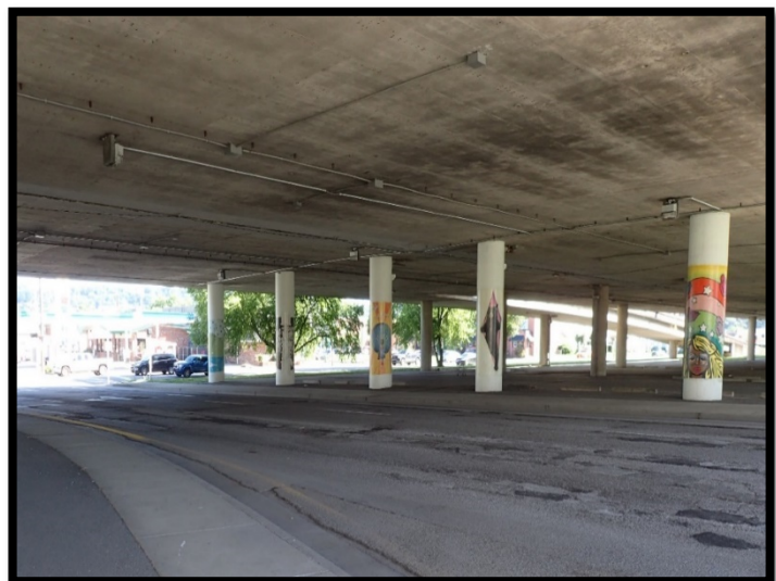
Photo 3: Damaged Pavement Under I-64 Interstate
