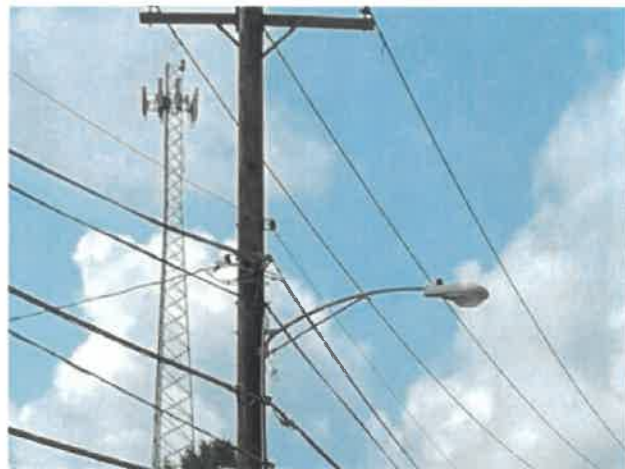
Existing cobra-style lighting in Town of Belle
