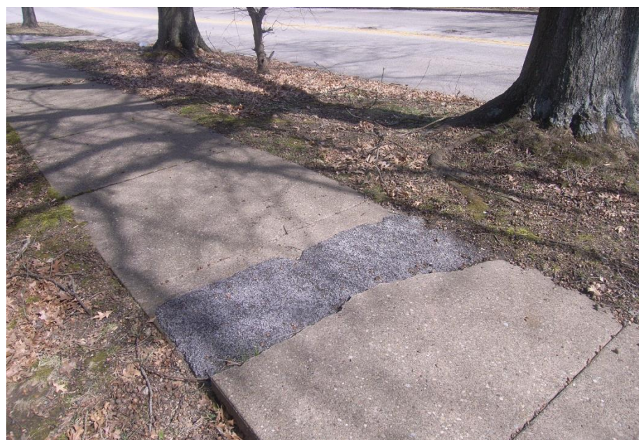
Figure 5-12: Uneven Sidewalk along Third Street near Kanawha Terrace
