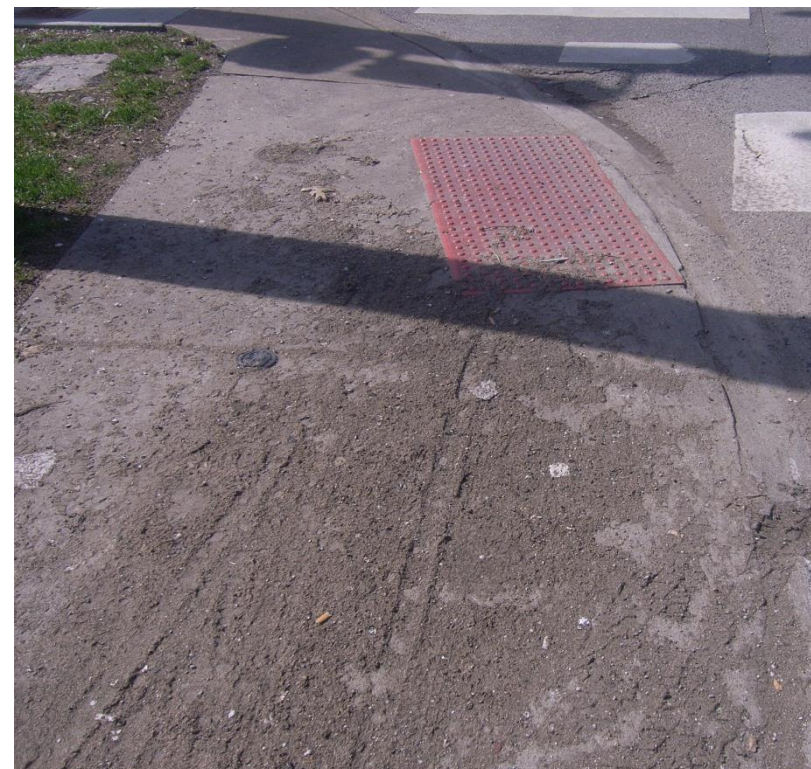
Figure 5-11: Gravel and Dirt on Sidewalk at the Third Street and MacCorkle Avenue Intersection
