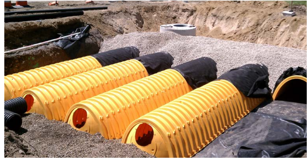
Example of an underground stormwater detention vault allowing the greenspaces to be accessible for passive recreation.
